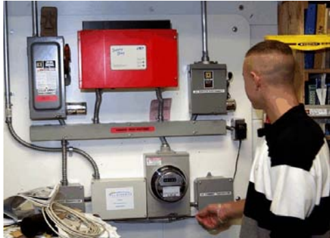
Figure 15. The inverter and related equipment are installed in a secure electrical room.
