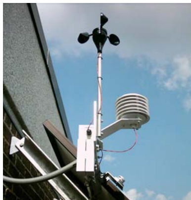
Photo Credit: Solar Works, Inc.
