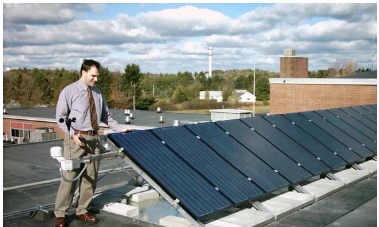
Photo Credit: Solar Works, Inc.
