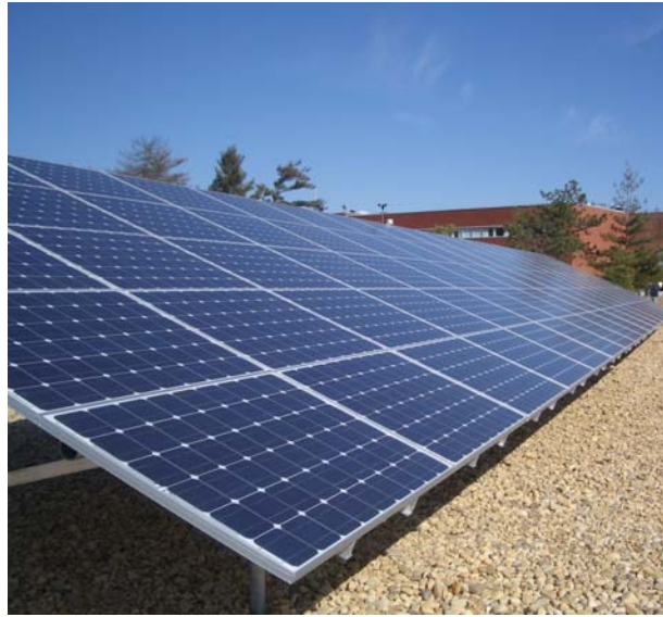
DuPont photovoltaic installation
